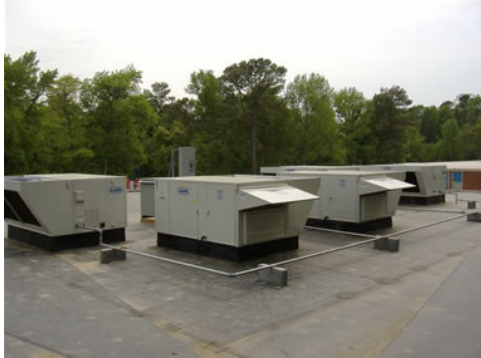
Typical Air Handler Units
