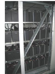
Uninterruptible Power Supplies
