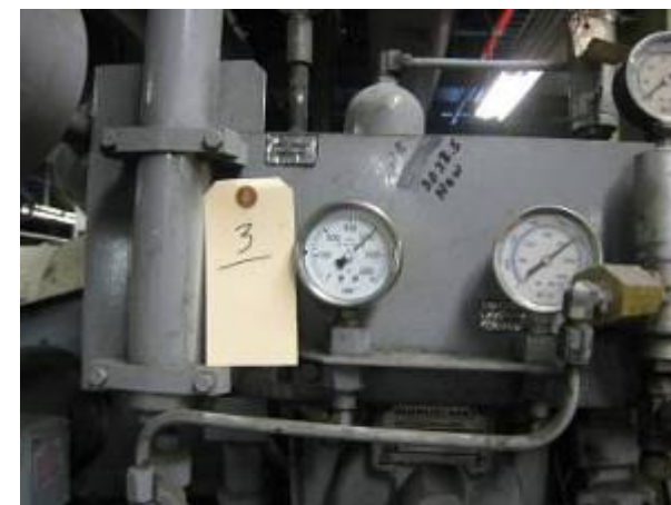
Hydrogen Dryer Tower Pressure
