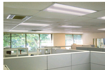
Legacy Fluorescent Lighting
