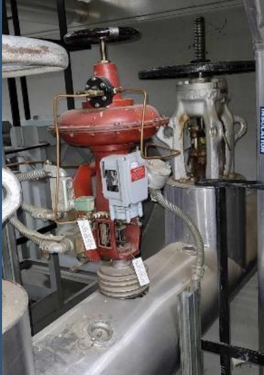
Valve Cycle Isolation Monitor
