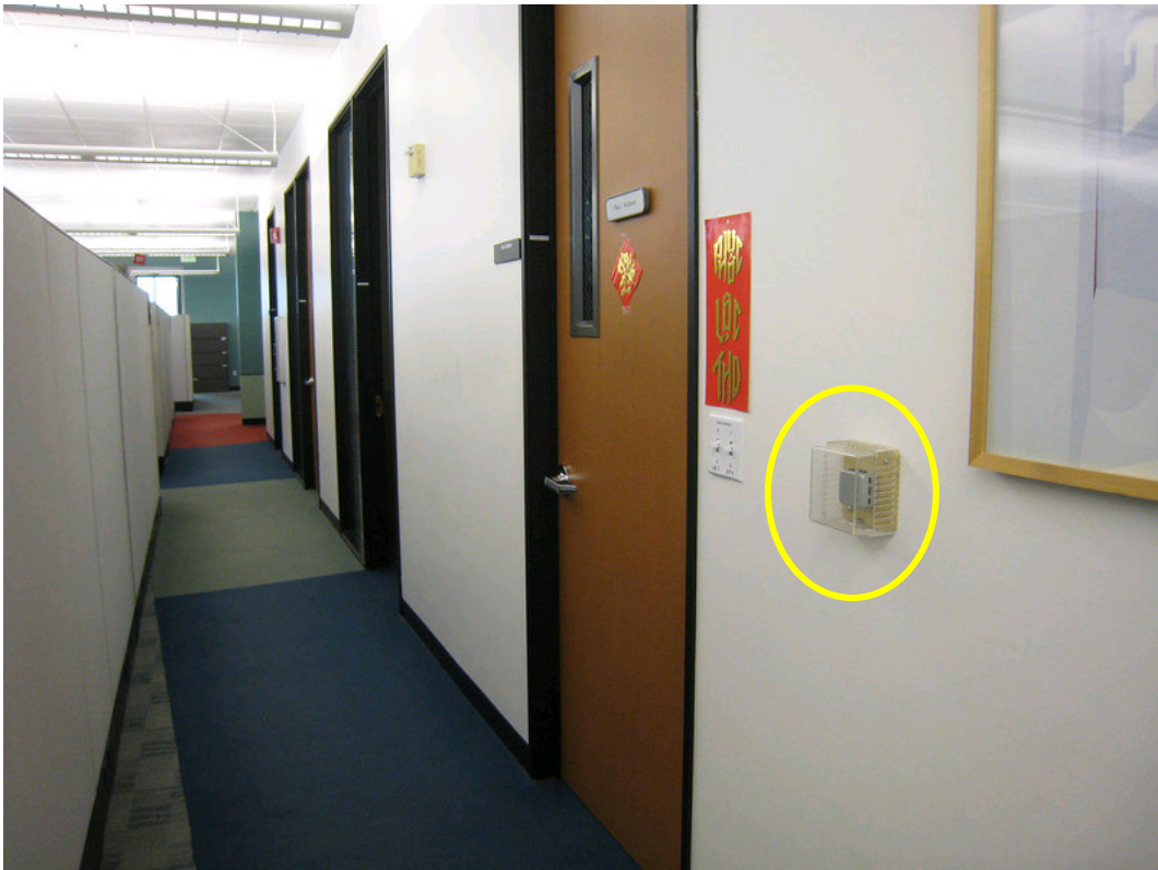
Figure II – Existing Pneumatic Thermostat prior to retrofit
