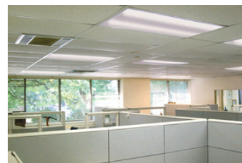
Legacy Fluorescent Lighting
