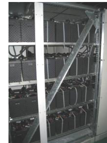
Uninterruptible Power Supplies
