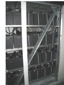
Uninterruptible Power Supplies
