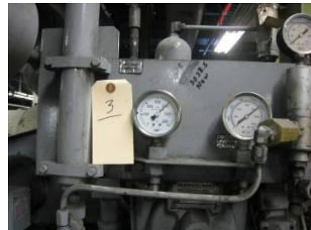
Hydrogen Dryer Tower Pressure
