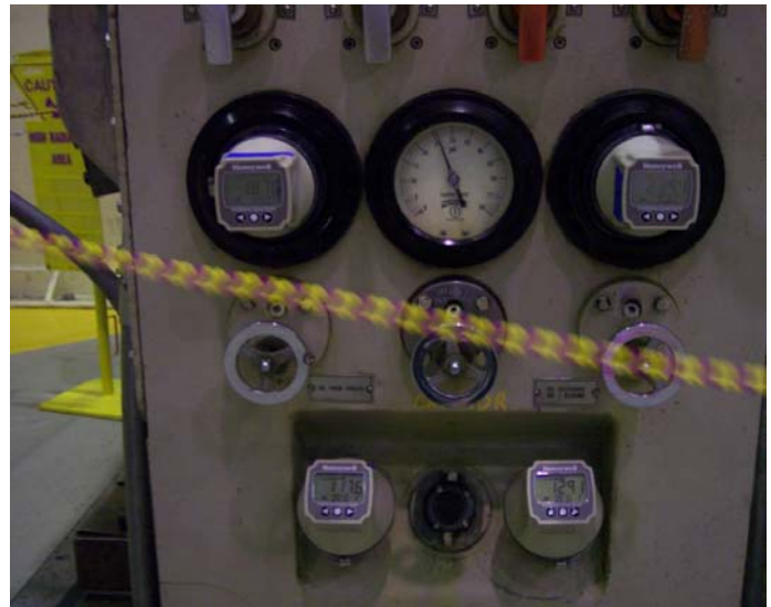
Honeywell Wireless Gauge Readers installed on gauges at the Vermont Yankee nuclear power plant.
